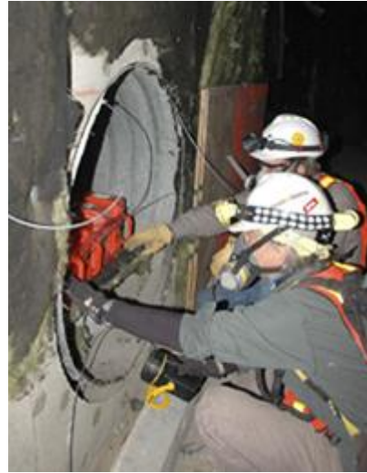
NIST electrical engineers Chris Holloway and Galen Koepke place transmitters in a protected air vent at the old Washington Convention Center prior to the implosion of the building.
